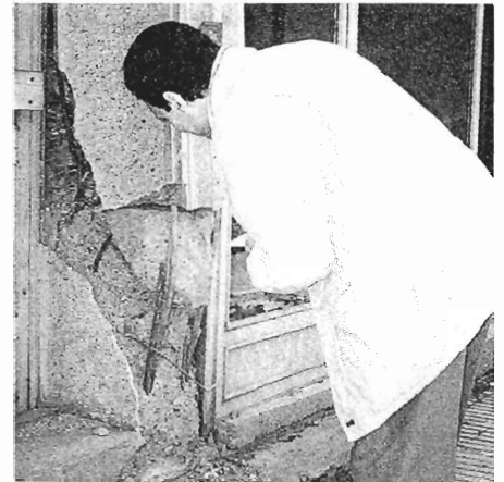
Above: Shear failure in a 3 storey RC building in Erzincan.
